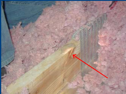
Bottom Chord Partial Fracture
