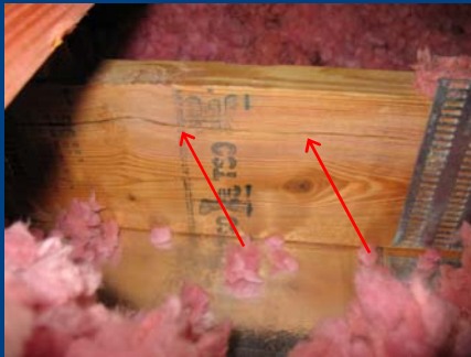
Bottom Chord Split
